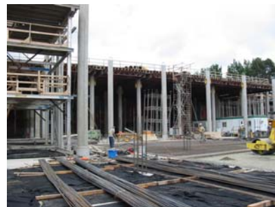
Little Mountain Reservoir
